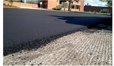
The milled surface is rough, but driveable, and is ready to be overlaid.
