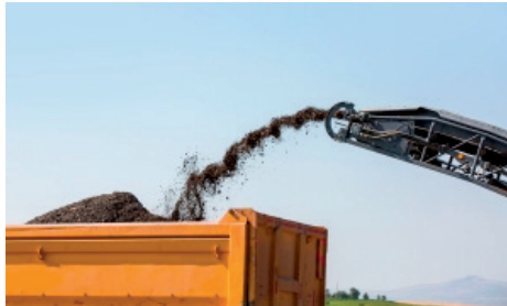
The old asphalt is passed through the milling machine and fed into a dump truck.
